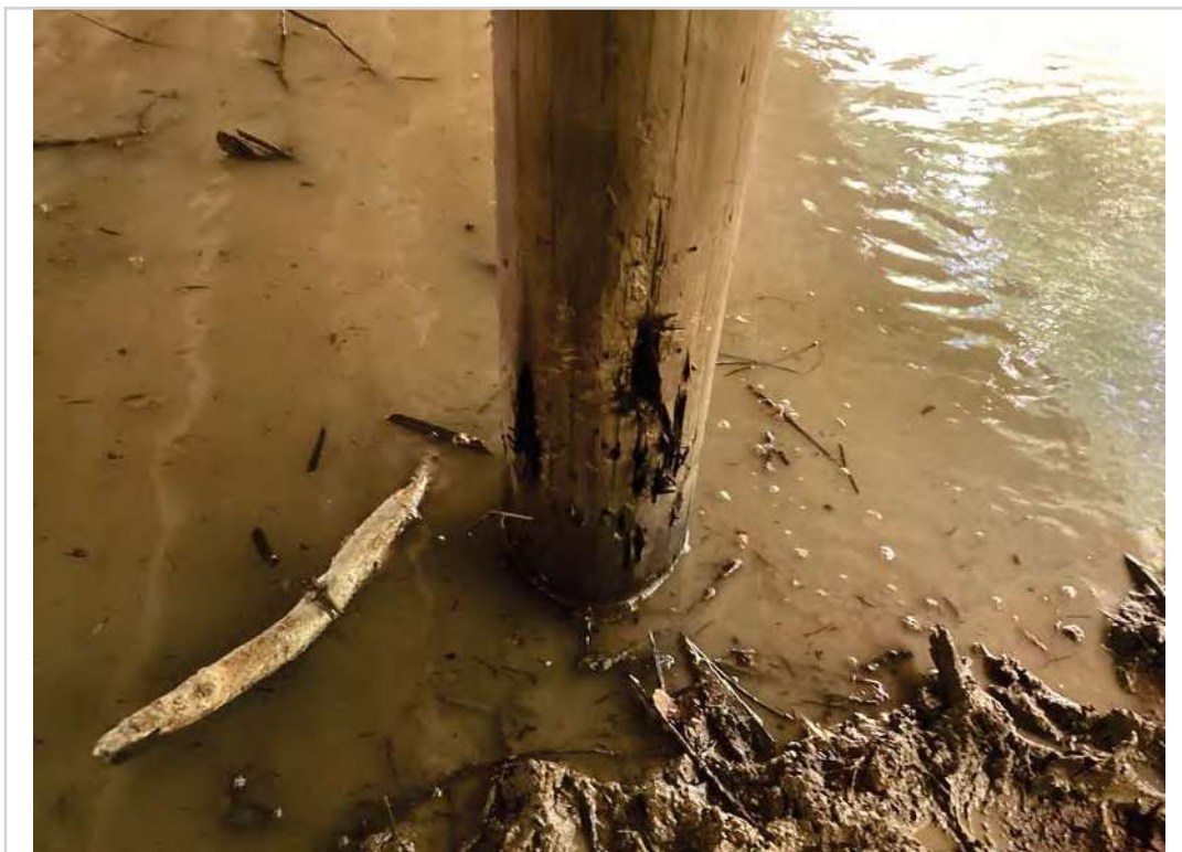
Bent #2 pile B decay
