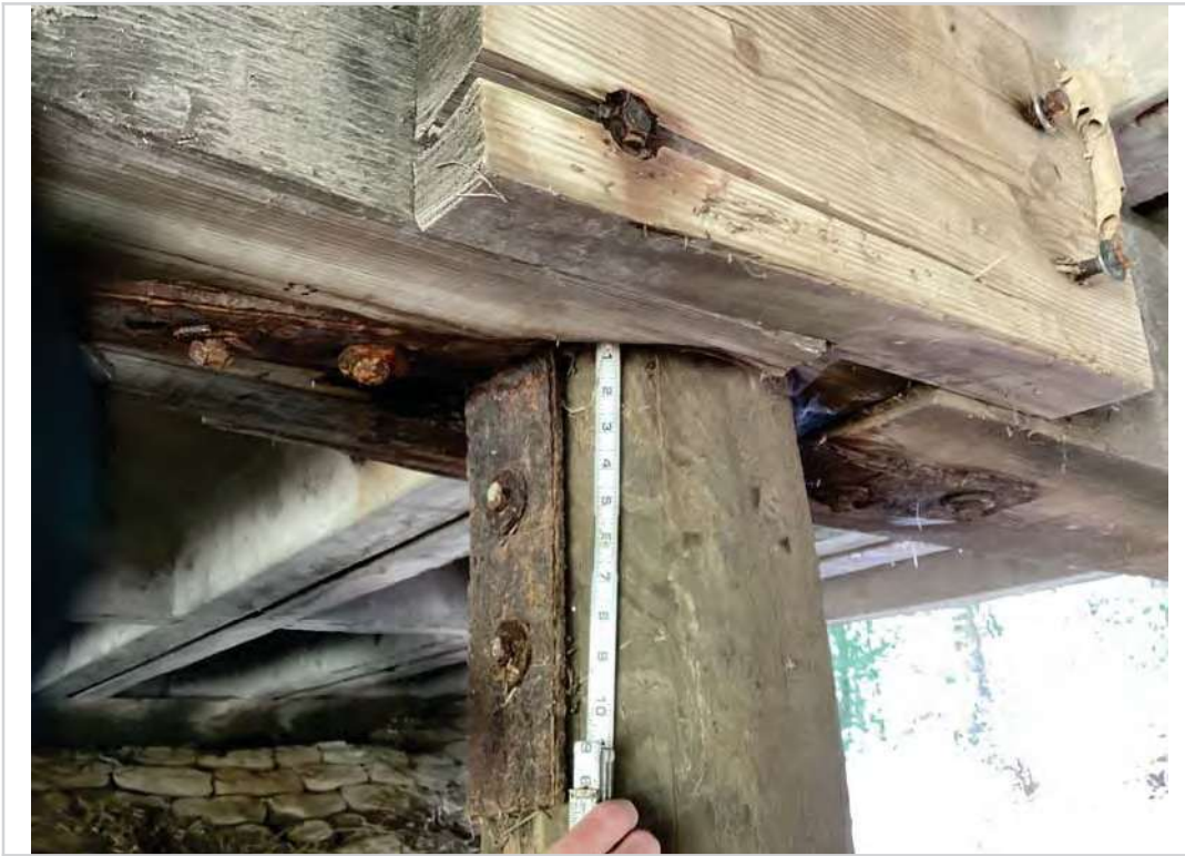
Bent #2 pile C impacting cap
