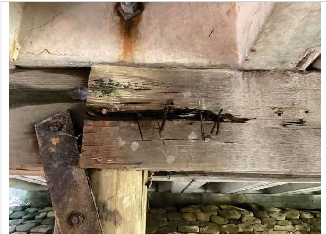
Decay/split, bent 1 cap rear
