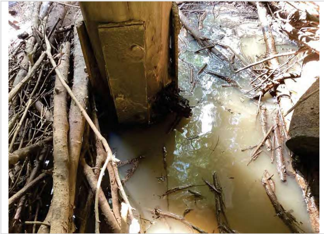
Bent #2 pile D decay
