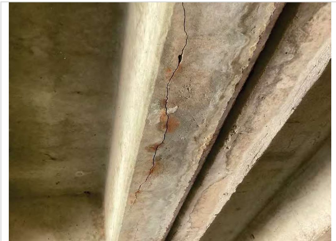
Span 2 slab C 1/16" cracks
