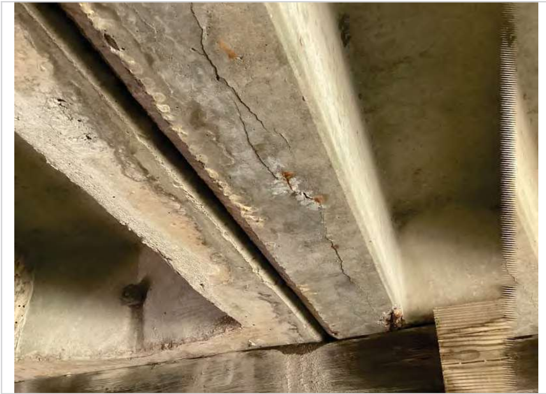
Span 2 slab C spall to steel
