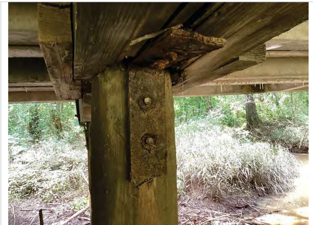
Bent #2 splice plates corroded (typical)
