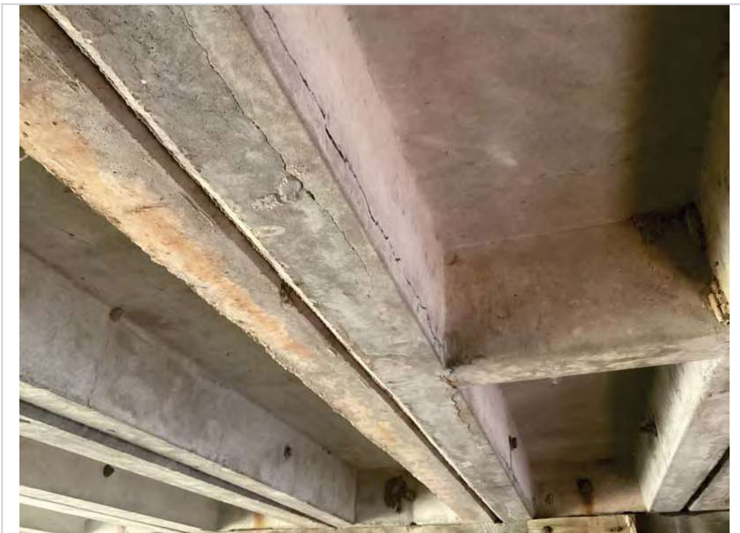
Span 2 slab E impending spall
