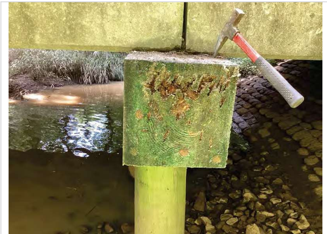
Minor decay, left end of cap, bent 1
