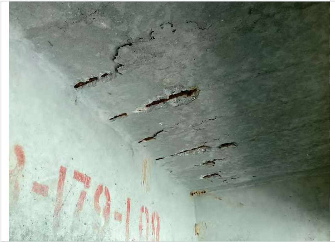
Span 1 slab A spall to steel
