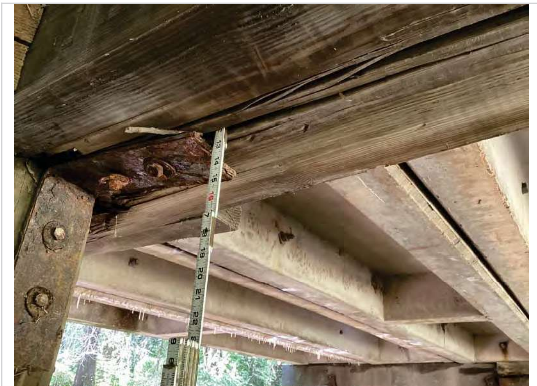
Bent #2 cap split all the way through
