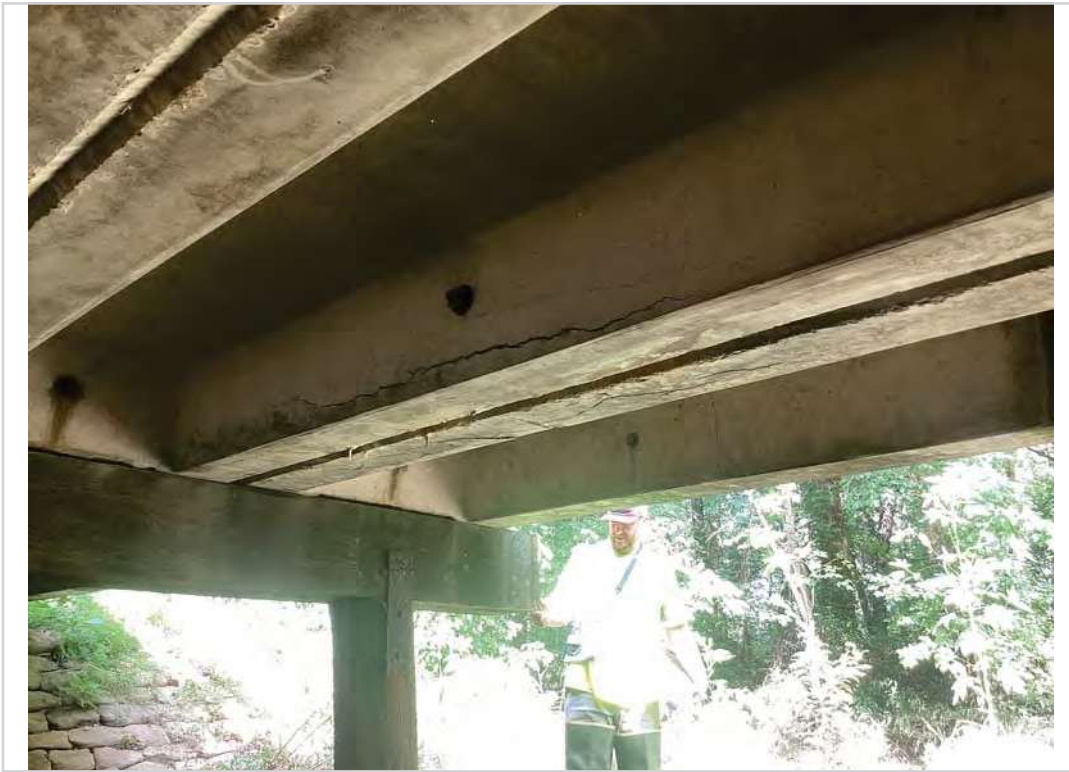
Span 2 slab B impending spall
