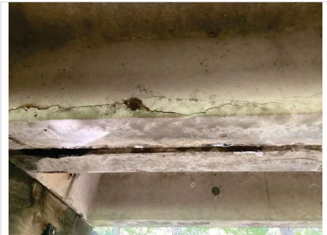
Span 1 slab F 1/16" cracks
