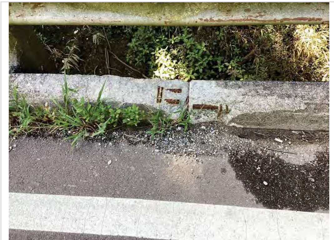
Spans #2&#3 right curb spall to steel
