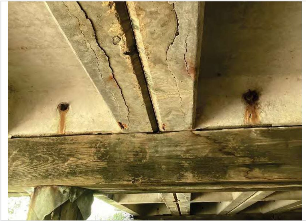
Span 2 slab A,B,C span connectors corroded and missing nuts
