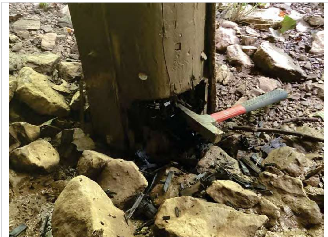
Decay section loss, pile A rear bent 1.
