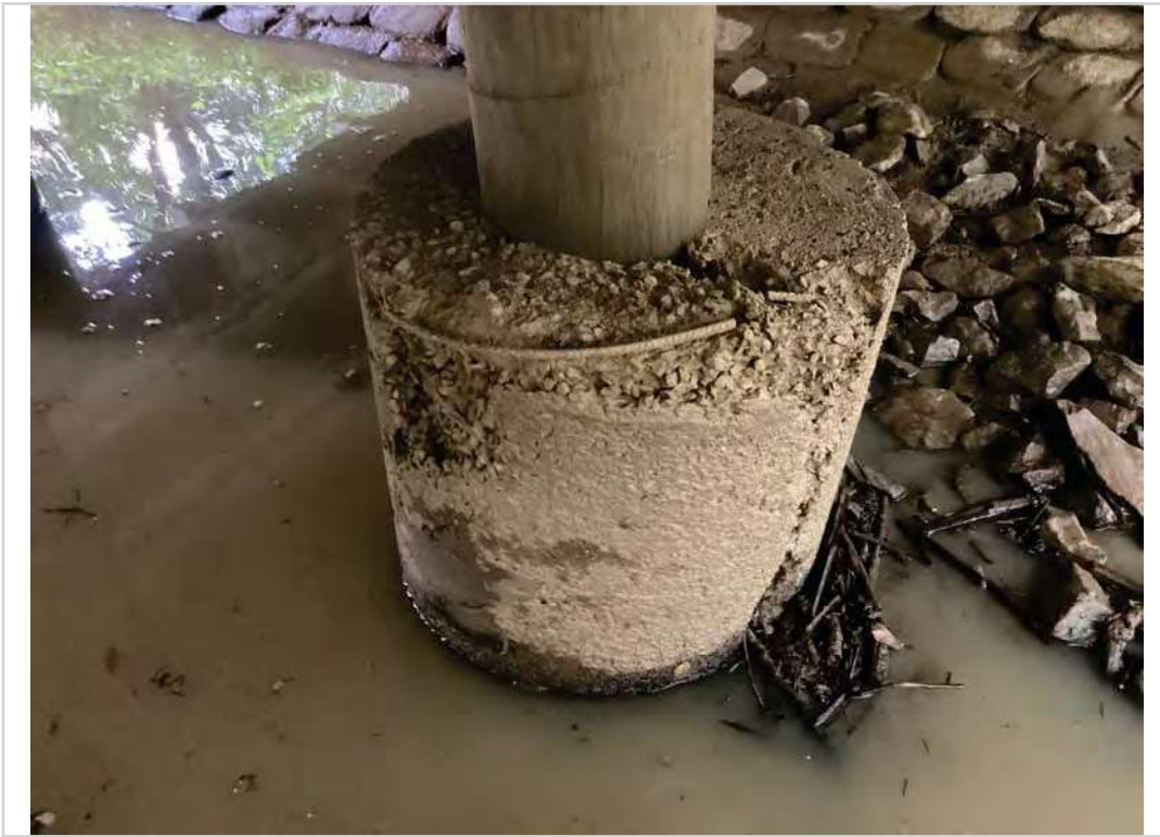
Spall to steel concrete casing, bent 1
