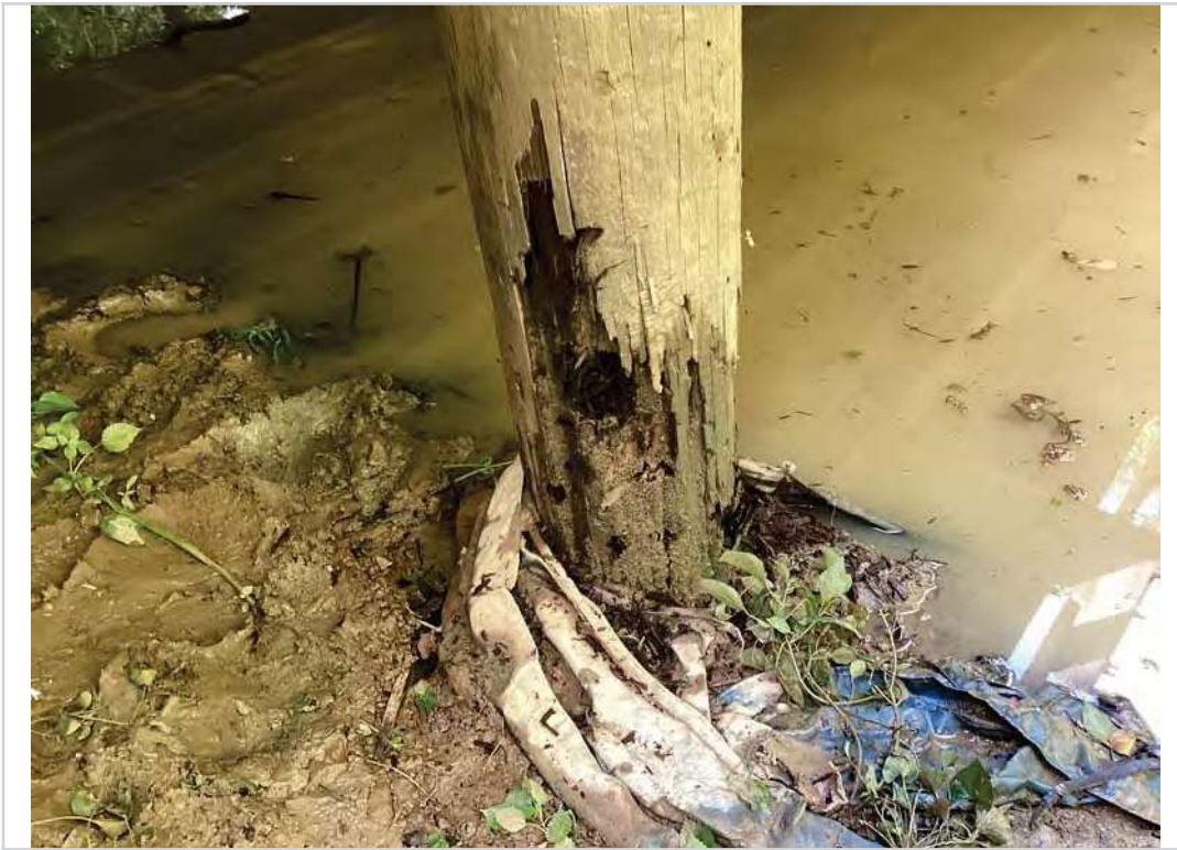
Bent #2 pile A decay
